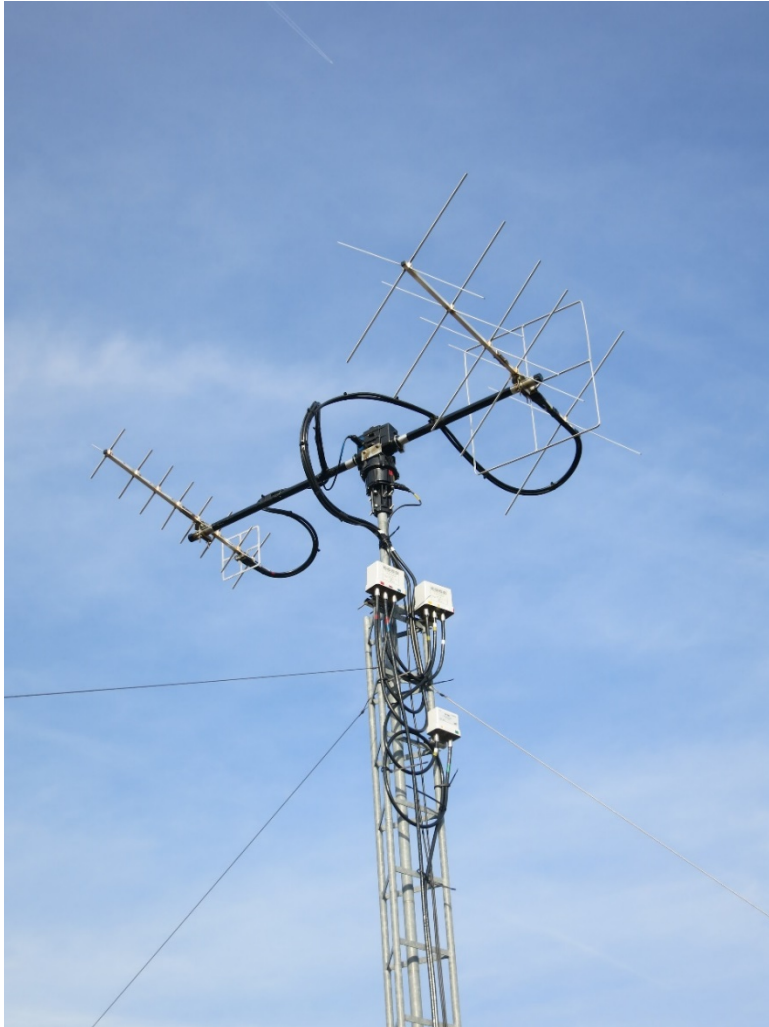
Satellite tracking antenna
