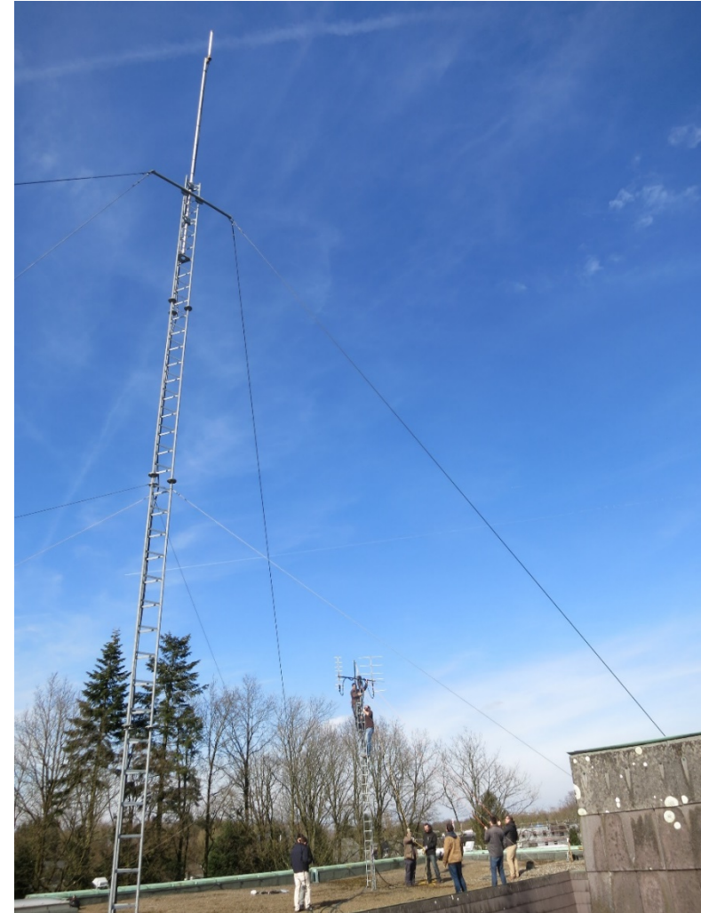
D-STAR repeater antenna
