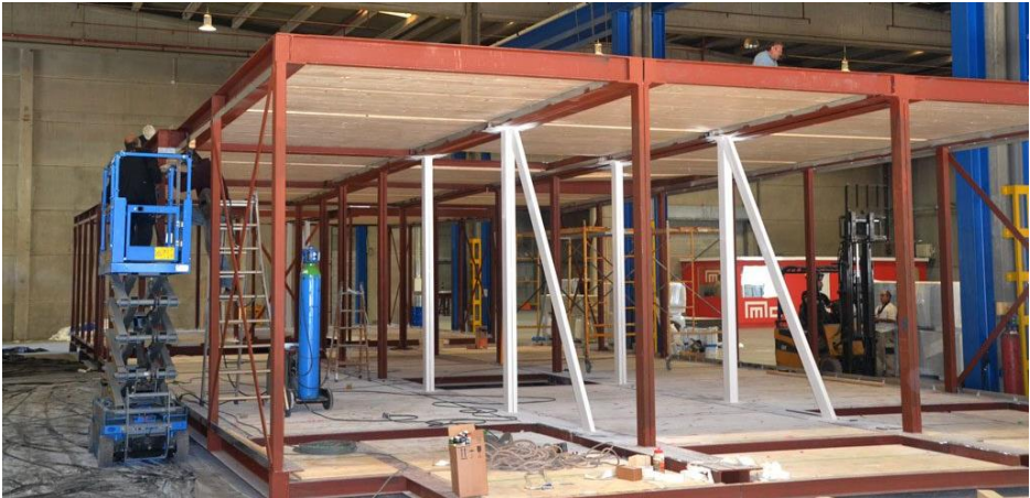
Figure 17: Offsite 3D modules manufacturing at Mothership, Barcelona © La Casa por el Tejado
