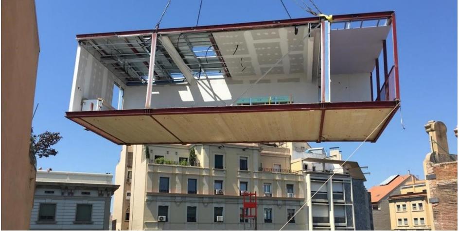
Figure 16: Lifting 3D modules over the rooftop in Barcelona © La Casa por el Tejado
