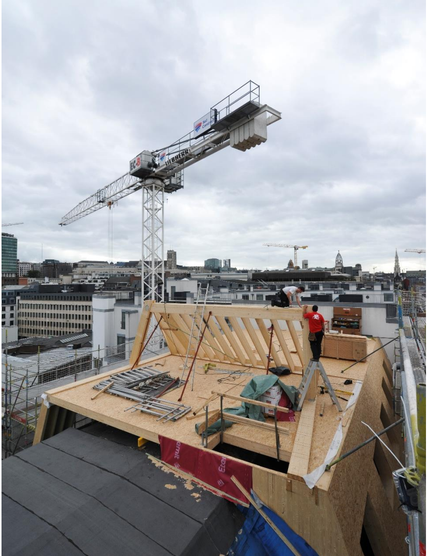
Figure 1: Sleep well in the sky hostel Project, Brussels, Belgium © Atelier d'Architecture Galand
