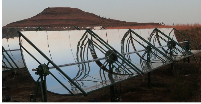
Figure 2.2: STG's parabolic trough collectors, installed in Lesotho [3]
