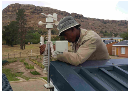
Figure 4.1: Weather station being installed on the roof of a typical clinic in Lesotho
