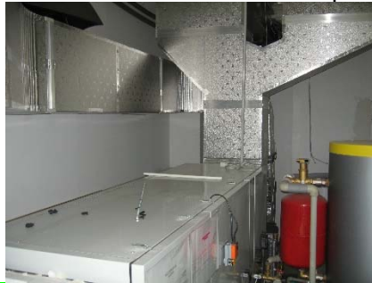
Figure 3.6.2: Ventilation system and the Heat recovery unit (HRU) of PH AMVIC
