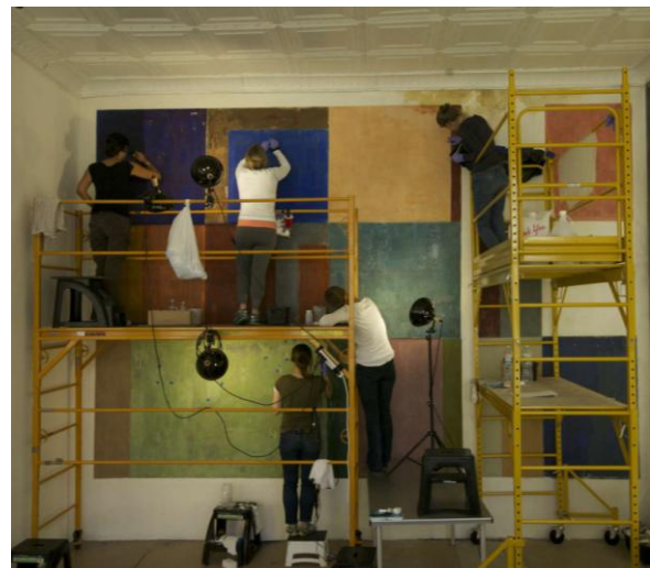
During treatment. The oil stain is visible at the top
